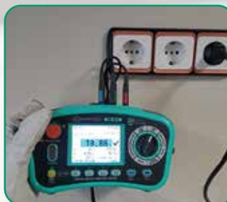
Loop test from a wall socket
